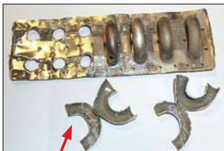
Image 3 Image reveals a cutaway section of the U-bends. There are visible signs of foreign matter collected on the inner walls of the U-bends.
