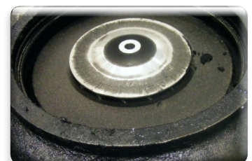
Compressor end oil leakage
